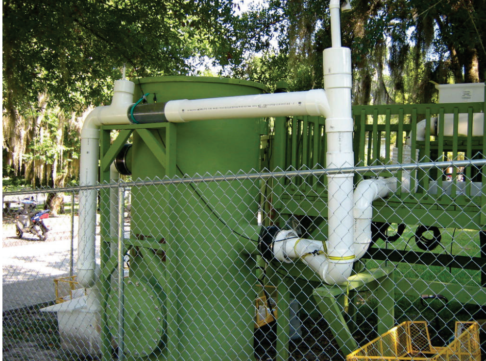
Figure 6 Photo of field test set-up for the Jellyfish ® Filter JF4-2-1. Below-deck inlet pipe enters the right side of the vessel and outlet pipe (invert at deck level) exits the left side of the vessel. External bypass piping has invert of horizontal section 18 inches above deck level.
